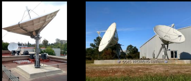
Typical GRB Receiving Antennas
